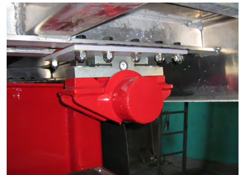
Hinge Pin Loadcell Installation
